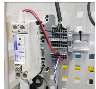
(12) 24 VDC power unit (provided by customer)
